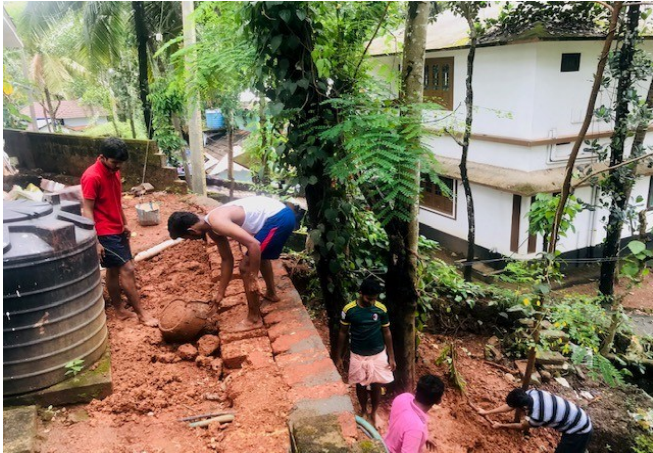
Volunteers of the unit are taking part in the compound wall construction of a needy family at Veidyarangadi, Ramanattukara.
